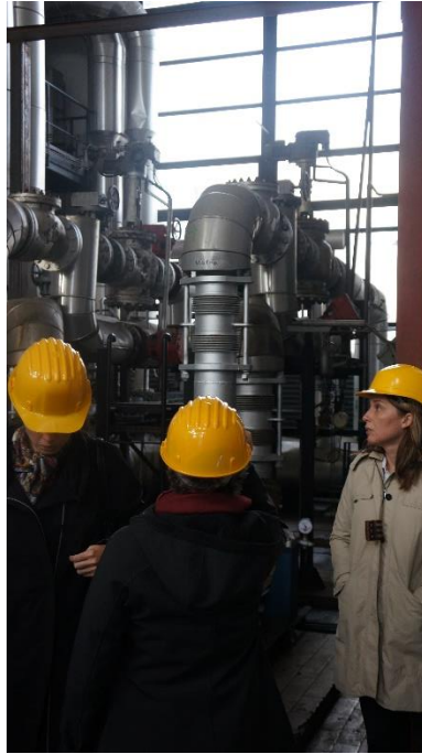
In the facility of the District Heating Karlovac Ltd.
