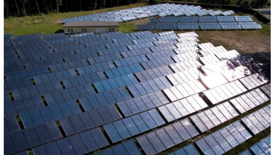
SDH - Waterworks Andritz, Graz; 2855 m 2
